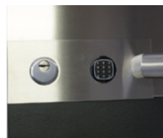
External keypad/card reader external lock
